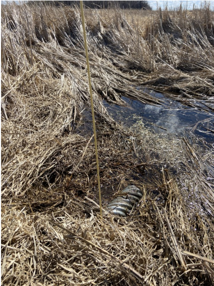
Left: Drain tile outlet
